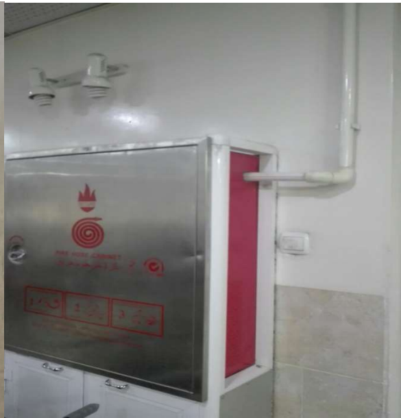
PPR pipe used
