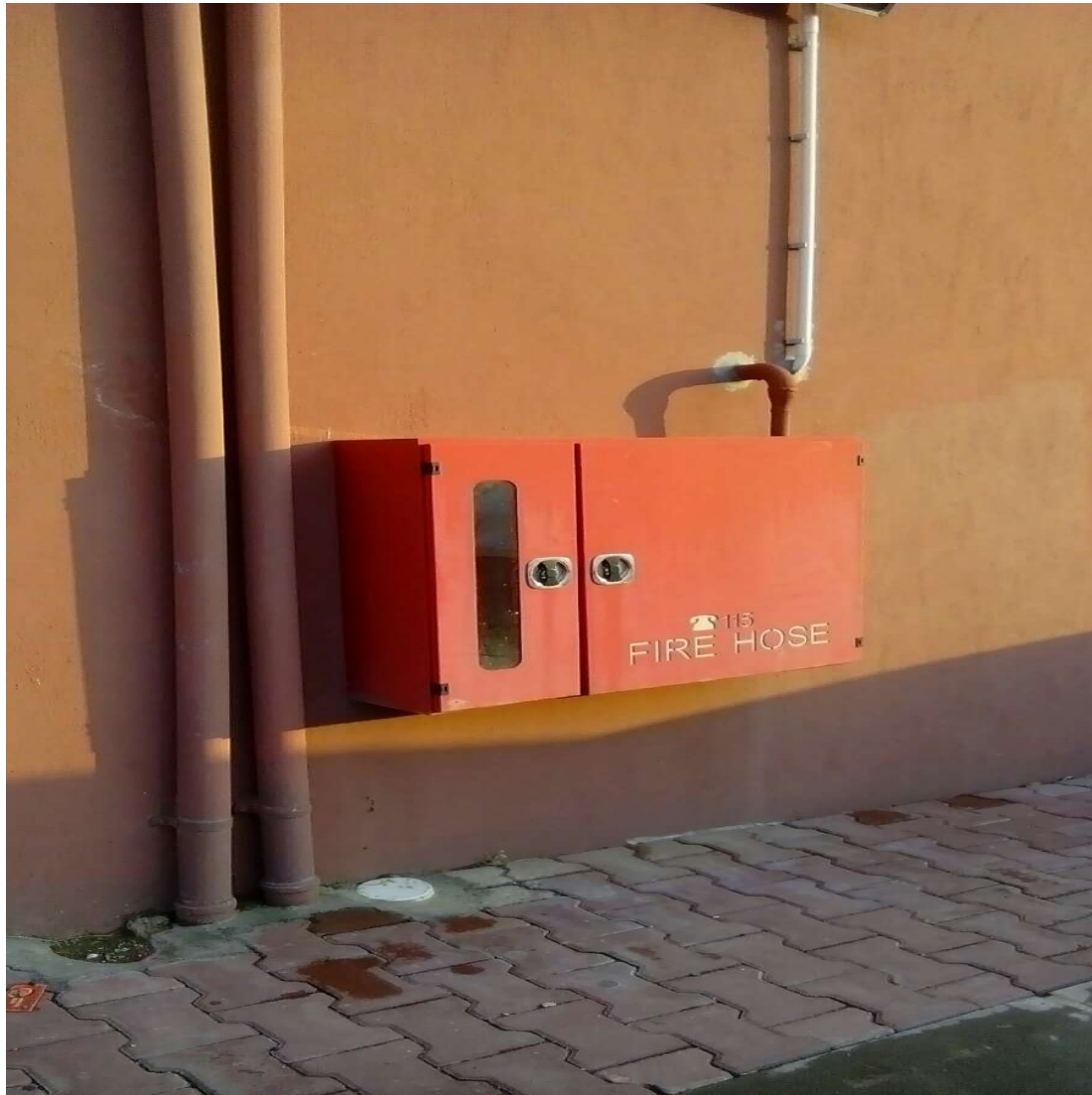
Wrong location of the stand pipe
