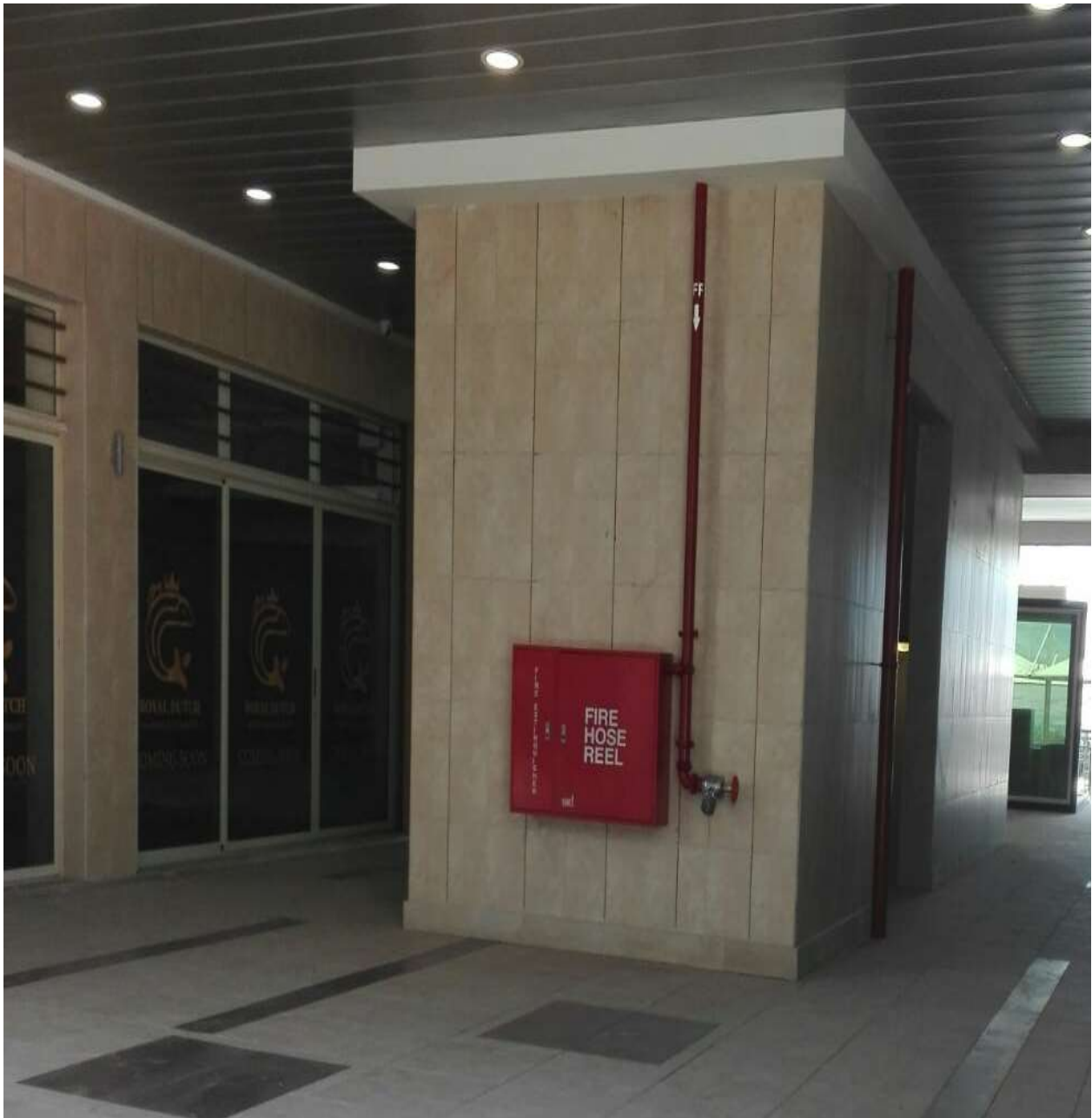
This Installation of FHC and fire department connection.
