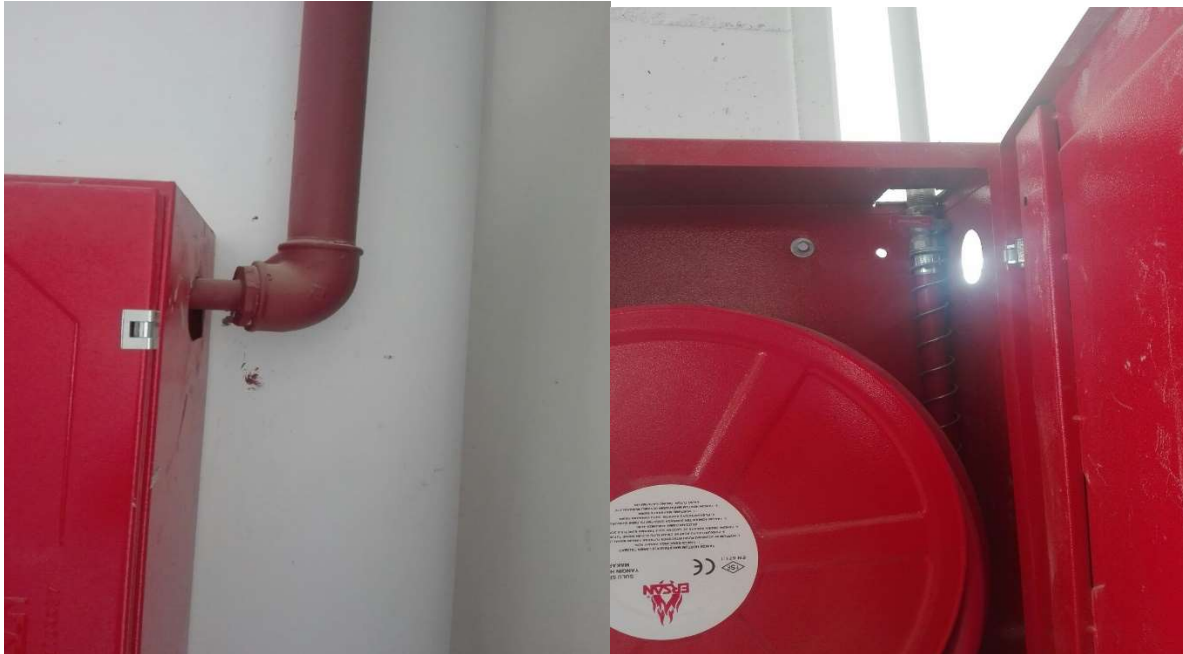
Wrong pipe size, over size branch
