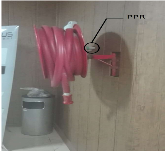
PPR pipe used
